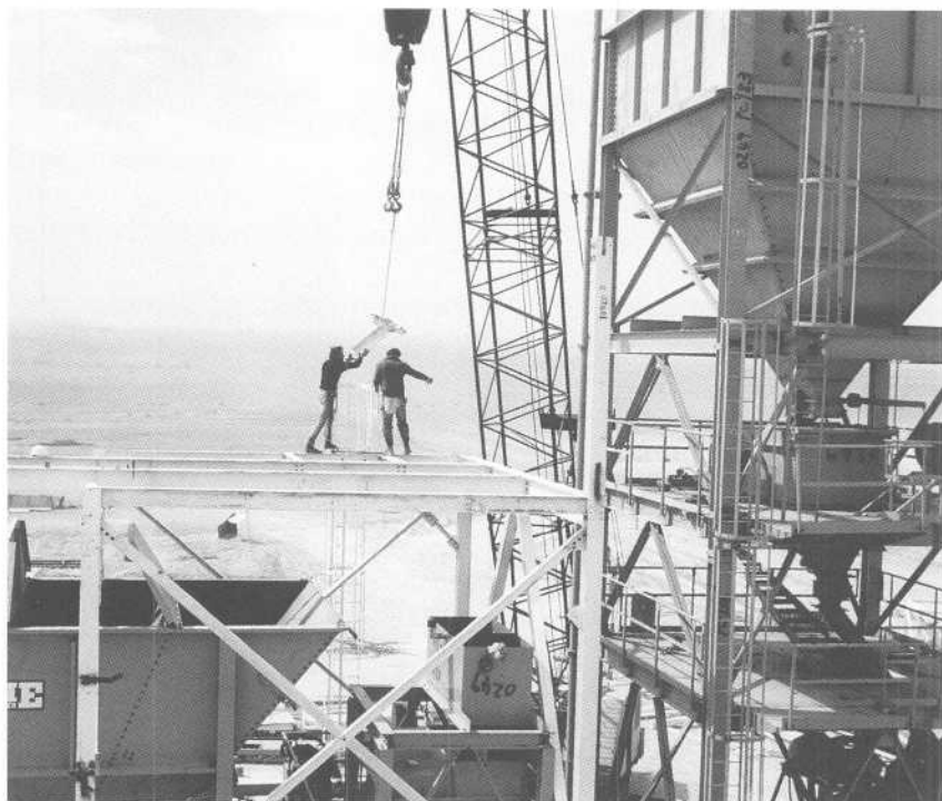
Bulk cement storage facility under construction at Ovda in the spring of 1980.
